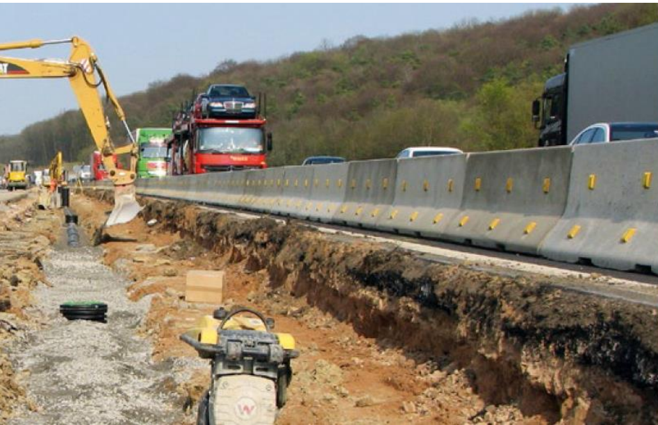
Installation in the cramped confines of a medial strip with moving traffic
