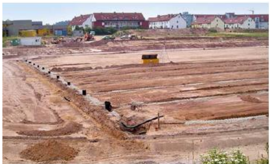
Example of the arrangement of a playing field drainage (full-size pitch 105m x 68m) with GALABAU- inspect chambers at the narrow sides and EURODRAIN-PE/SIROPLAST-K drainage pipes
