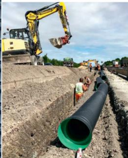
New construction of the carriageway in the direction of Ulm by storm water sewer pipe AQUATUB-Rw
