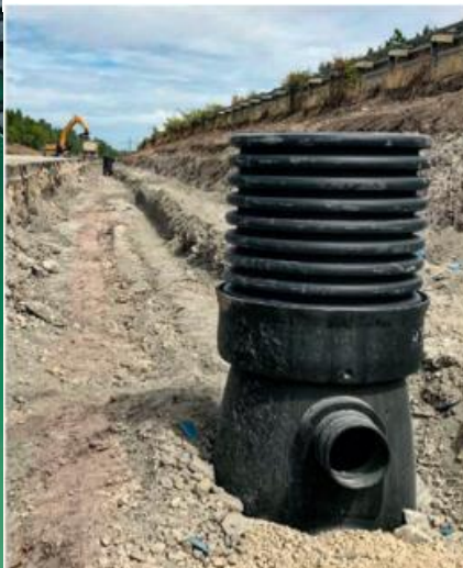
Drainage with the robust chamber system MULTI-inspect DUO prior to demolition of concrete surface
