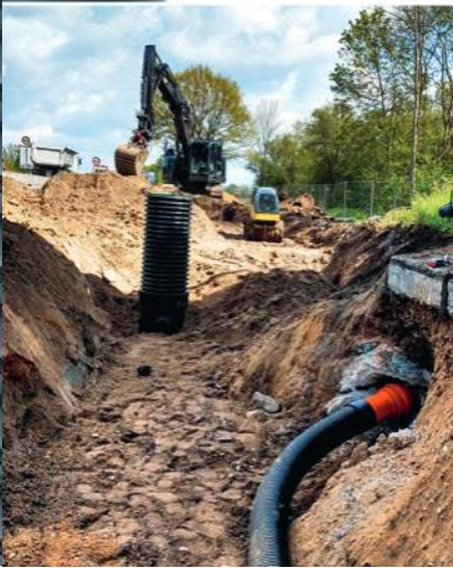
Connection of road outlets to the roadway drainage system at an elevated crossing
