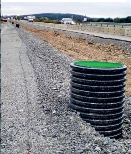
Extension of carriageway in direction of Nürnberg with drainage of medial strip
